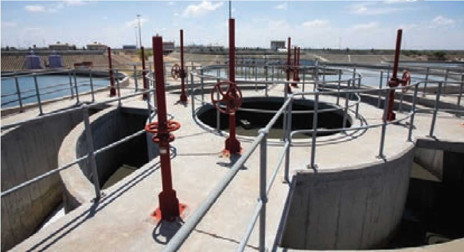
Gaborone Wastewater Treatment Plant
