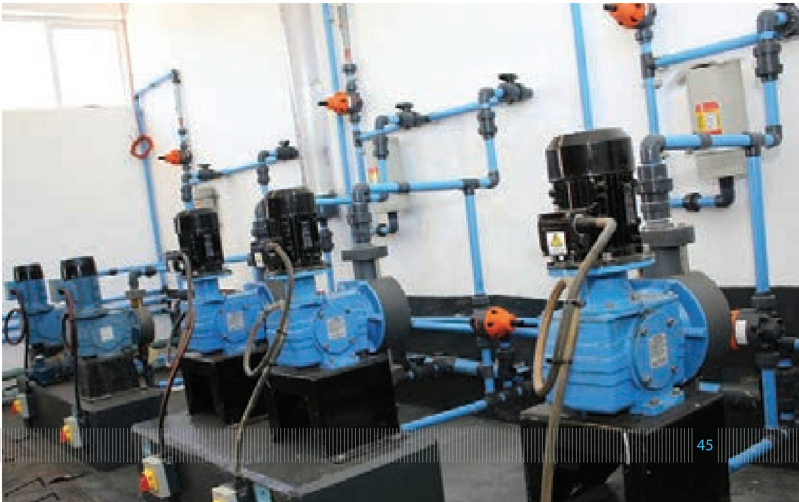
Chemical dosing room - Mmamashia Water Treatment Plant
