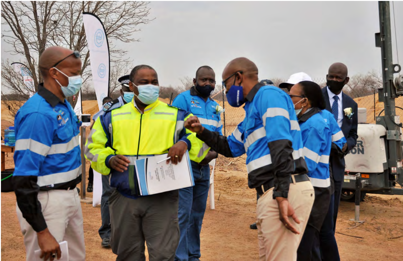
WUC Board Chairman, Mr. Noble Katse; Honourable Minister for Land Management, Water and Sanitation Services, Mr. Kefentse Mzwinila; and WUC CEO, Mr. Gaselemogwe Senai, during the groundbreaking of the Masama 100km pipeline.
